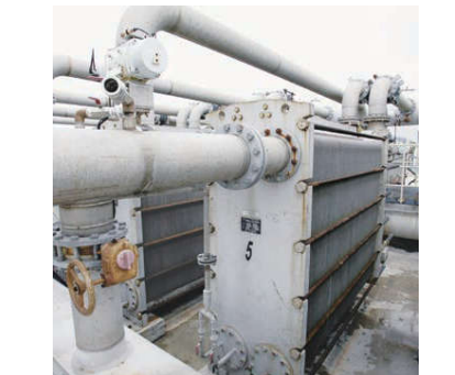
Heat exchange of black liquor / white water, oven blow gas condensation, waste heat recovery
