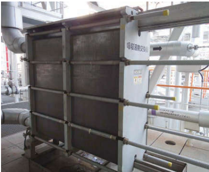
CO 2 recovery, desulfurization plant solution heat exchange
