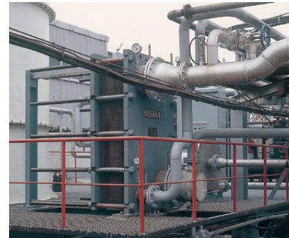
Solvent recovery, exhaust gas cooling
