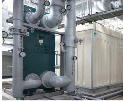
Heating / cooling system, water heating, district heating / cooling, building heat storage tank systems, unused energy
