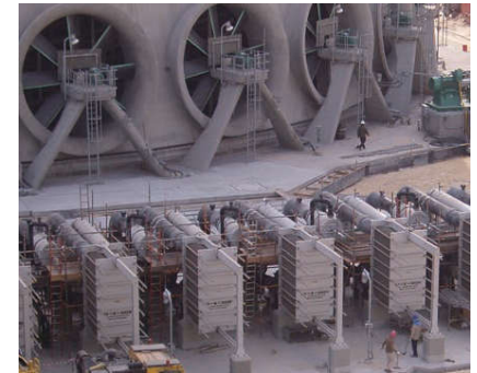
Central cooling system
